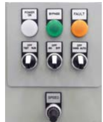
Manual Bypass controls
